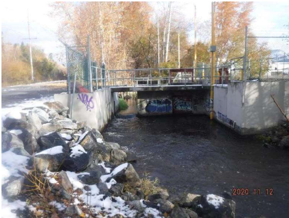
Appendix Photo 2. View (upstream) at the lower side of the diversion structure.
